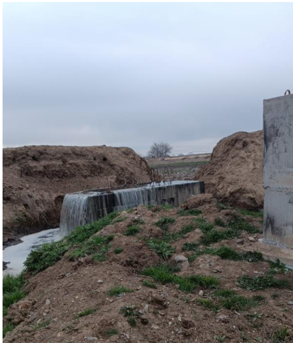
Figure 6. Observed wastewater discharge from collection pipelines in the project area (March 4, 2026)
